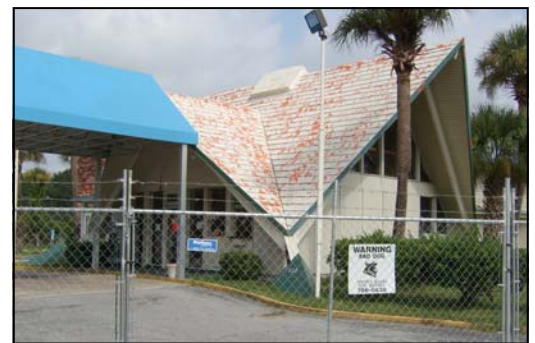
The Civista Inn on Golfair Boulevard has been shut down and represents a major community victory over slum and blight.
