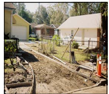
NJCDC inspires change on West 27th Street! This homeowner began installation of a new garage and driveway after an NJCDC home was built next door.
