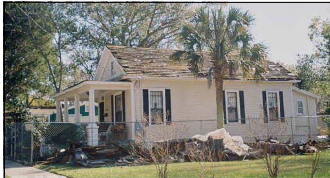
On West 30th Street, a homeowner replaces an old roof with a new one, adding to the beauty of the neighborhood.
